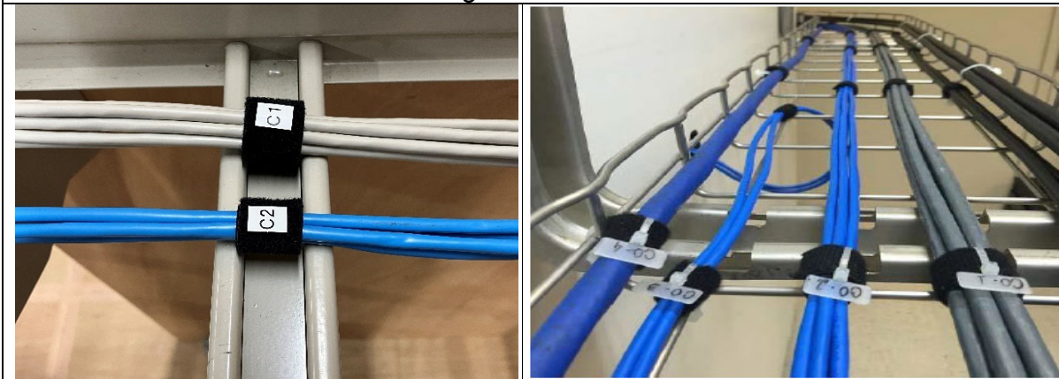
Labeling bundled cable (Not recommend).
